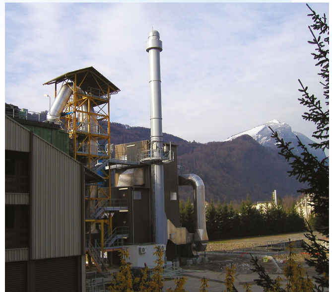
© Lühr Filter. Incinerator. Image reproduced with kind permission.
